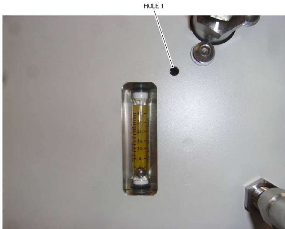
Figure 16 - Nitrogen flow meter
