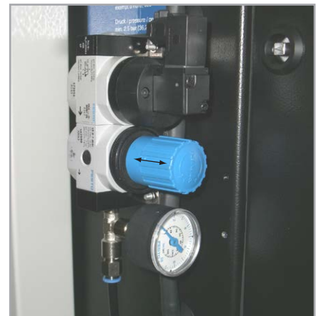
Fig. 5.7 Set up the pressure at the supply unit.
